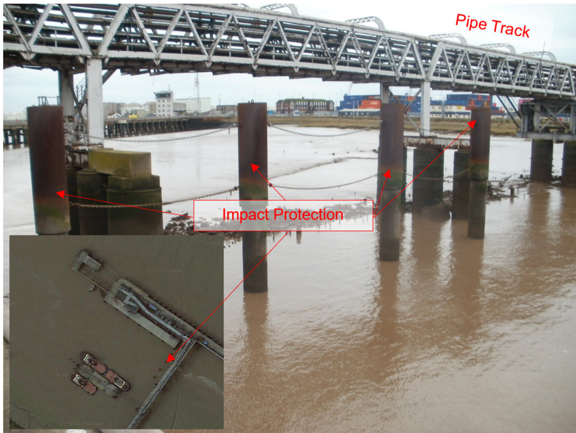
Figure 2: Impact Protection installed at Immingham West Jetty Berth 4 to protect pipe track.
